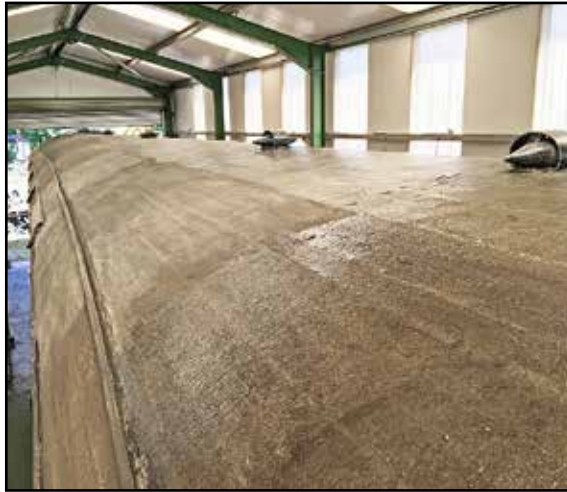
TTO 56856 has had its roof patch repaired and will now receive two coverings of Durashield. It is pictured with bonding primer applied. Photo: Paul Johnson.
