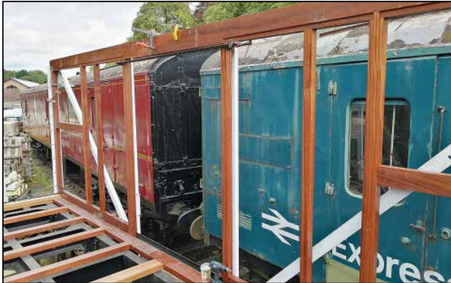
The first side of the Fish Van framing is erected. The two clamps at the top centre are holding the two half-sides together - there is a scarf joint where the two join. As Eric Morecambe would say - you can't see the join. Photo: Andrew Daniel.
