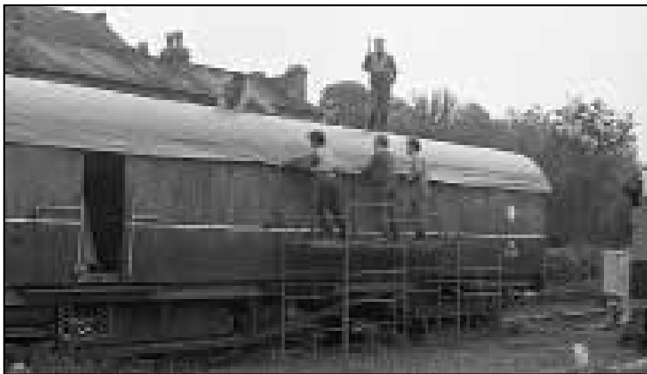
The year - 1984. A replacement roof sheet is being fitted. On the roof, left, is, Membership Secretary Peter Wilson, former guard Steven Bellamy, whilst on the tower is, left, Secretary Dave Cullingworth, former Chairman Roger Melton and Advisor, Andrew Daniel. Photo: Murray Brown.
