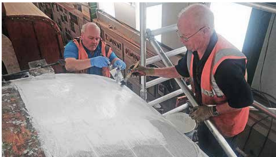
Durashield is applied to the polyester roof covering on TTO 23956 by Marcus Woodcock (left) and Ken Richardson. Photo: Gary Lyne.
