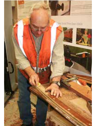
Mike Illingworth scrapes the old varnish of the curved cornice prior to revarnishing. This cornice is screwed onto the end of the carriage (23956) and traps the overhanging polyester roof covering. Photo: Murray Brown.
