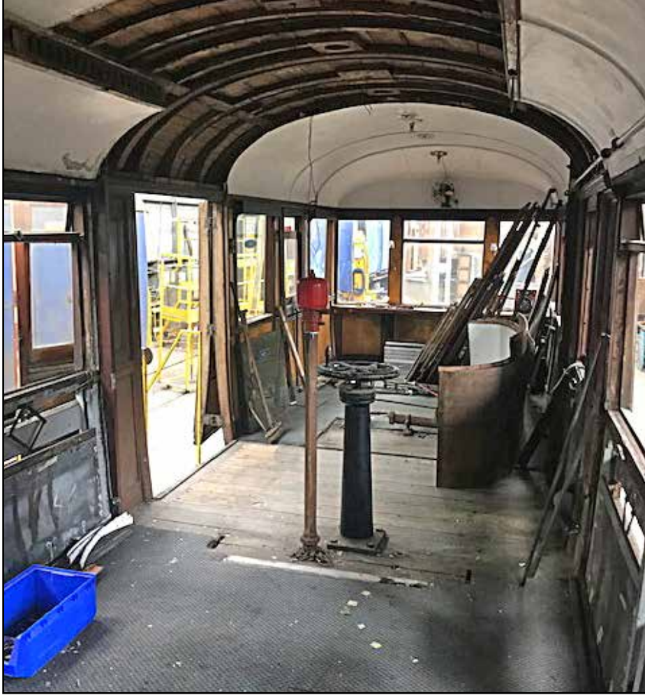
Work underway at Rampart, Barrow Hill, Staveley: The removal of the brake handle and brake handwheel will allow the entire space, seen here, to be given over to an observation area. Photo: Nick Stringer.
